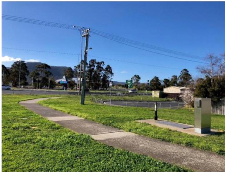
Figure 10: Existing TasGas infrastructure at end of McGough St in foreground with TasNetworks infrastructure, Brooker Highway & existing DEC in background
